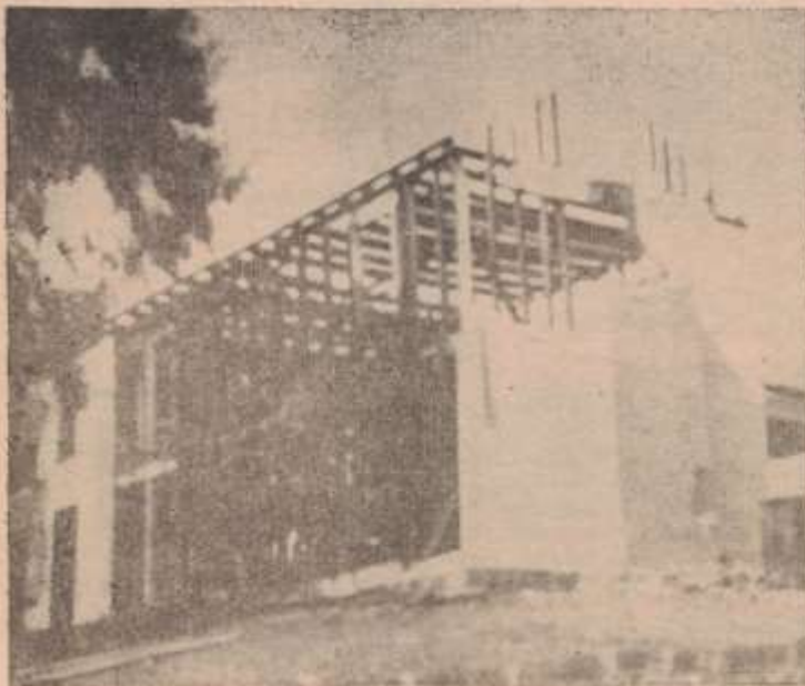
"AIN'T GONNA NEED THIS HOUSE NO LONGER" —Pictured above is the old Adair house on Main Street, one of the oldest homes in the county, being torn down. —Clarion Photo
